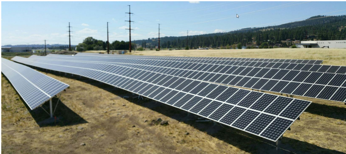
Boulder Park Community Solar Project
