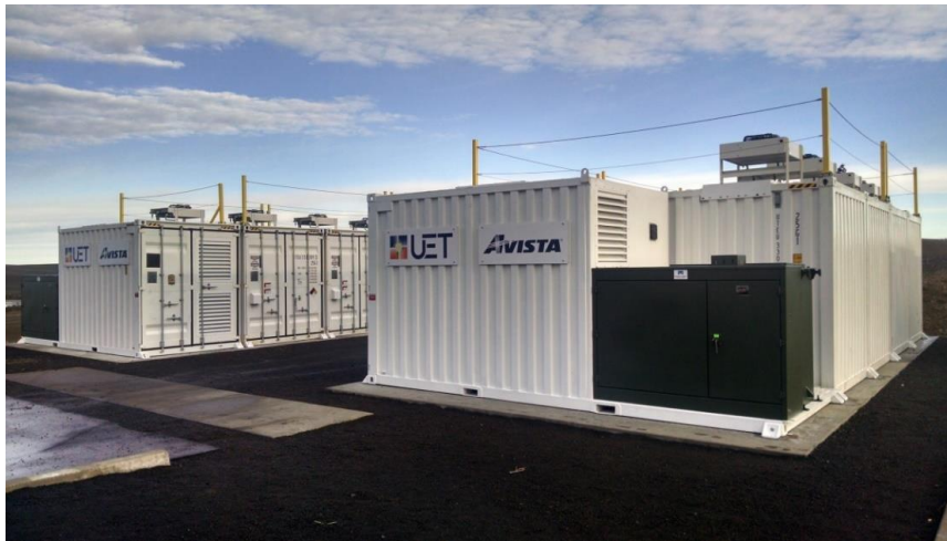
Turner Energy Storage Project, Pullman, WA
