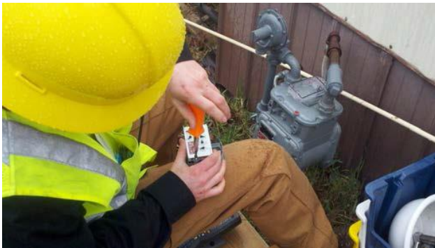
7 Retrofitting Natural Gas Meter Index with ERT
