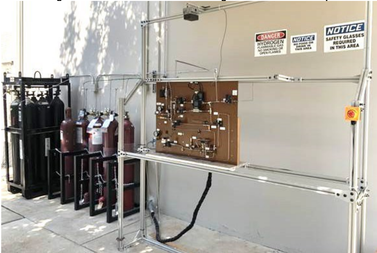
Figure 16: Controlled Gas Leak Testing Instrumentation Setup
