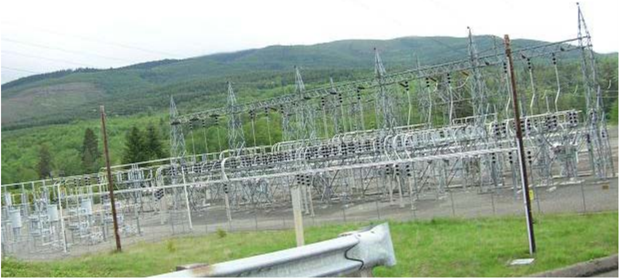
Figure 2-4. BPA's Fairmount Substation.
