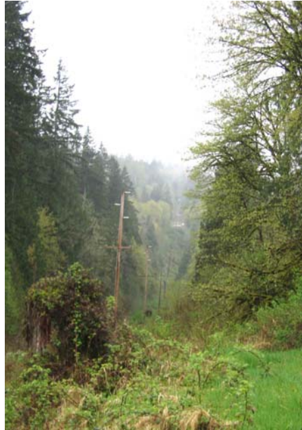
Exhibit 14-4: Vegetation Impeding ROW Access
