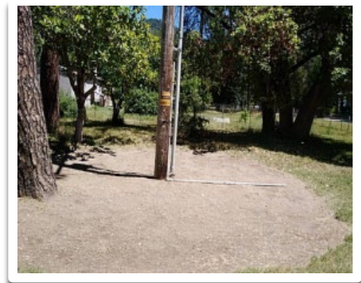
Figure 36: Pole Clearing at Pole Base
