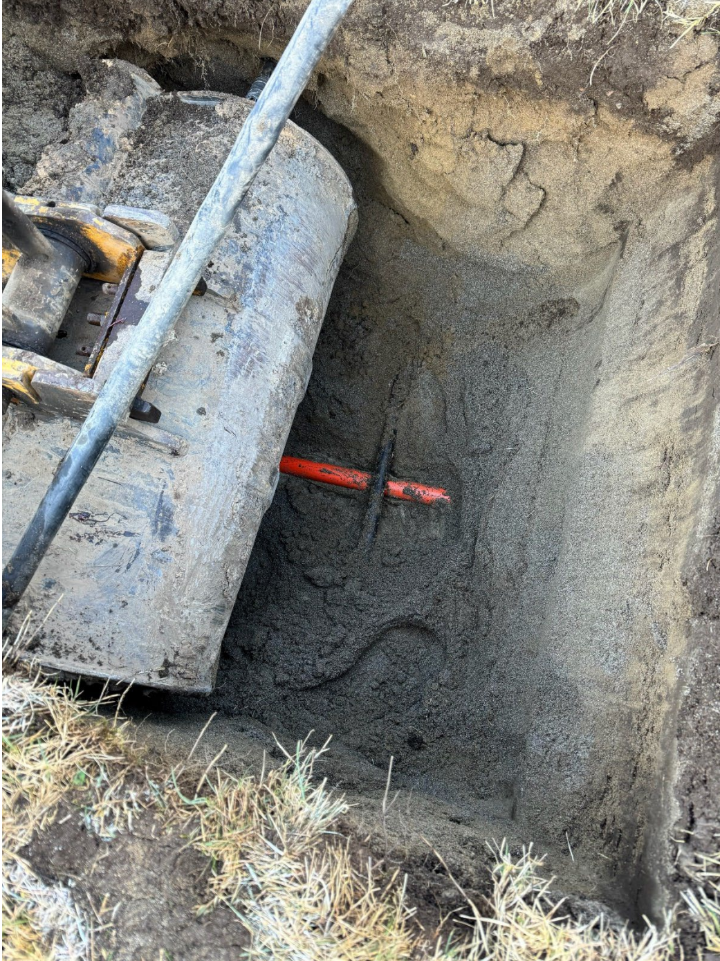
Figure 2 Damage above the service after hit by excavator bucket
