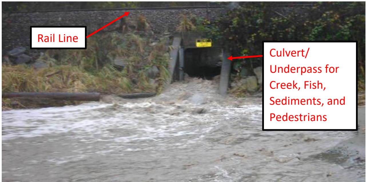
Photo 7. Flooding of culvert for pedestrian beach access – looking east from Puget Sound
