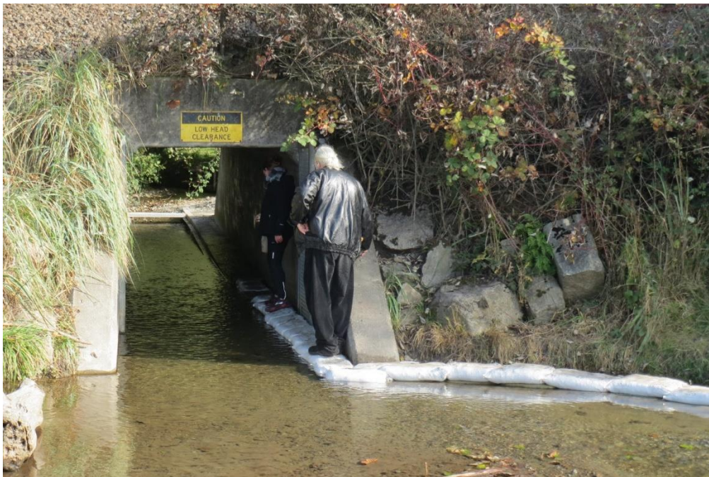
Photo 6. Low head clearance sign and sandbagged access below railroad tracks
