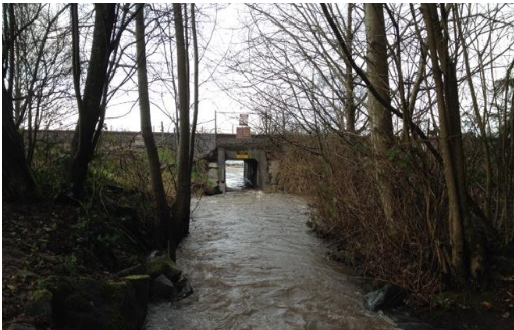
Photo 8. Flooded culvert for pedestrian beach access – Looking west towards Puget Sound
