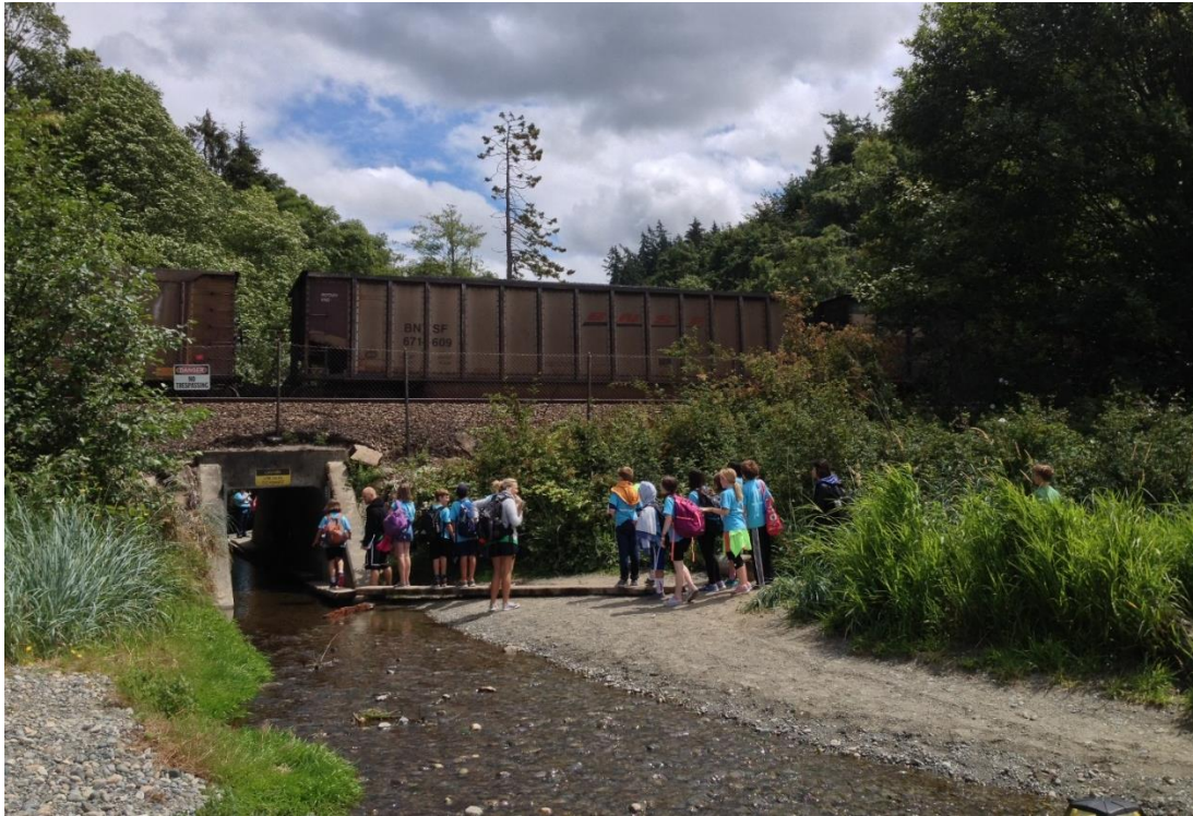
Photo 5. School group straddles ledge in culvert as grates are removed to accommodate fish passage (Existing Underpass)
