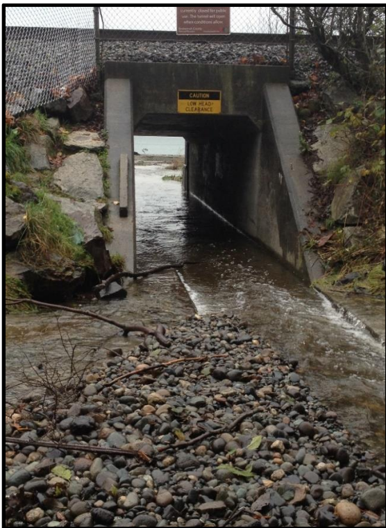
Photo 14. Sediment, critical for nearshore nourishment deposited upstream of the culvert doesn't easily reach the beach due to the barrier of the embankment and narrow culvert opening (looking east towards Puget Sound)
