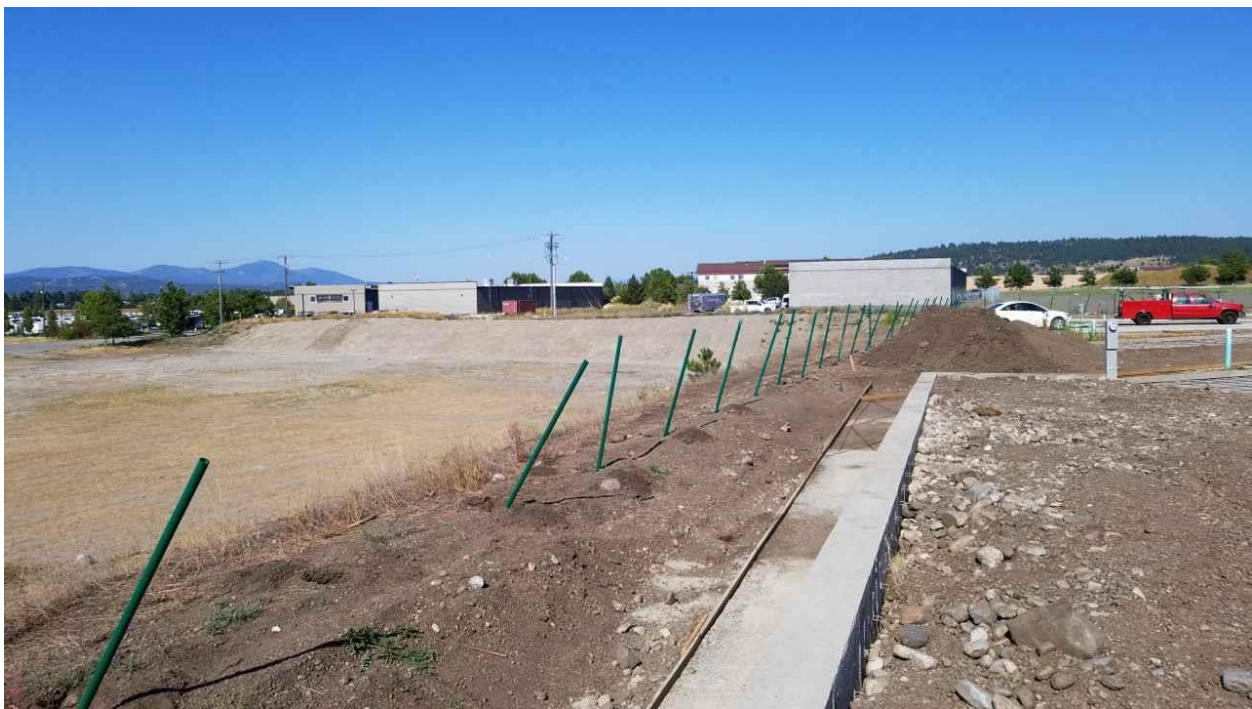
Attachment #6 – 3 Locator's pictures upon his arrival showing that post holes had already been augered
