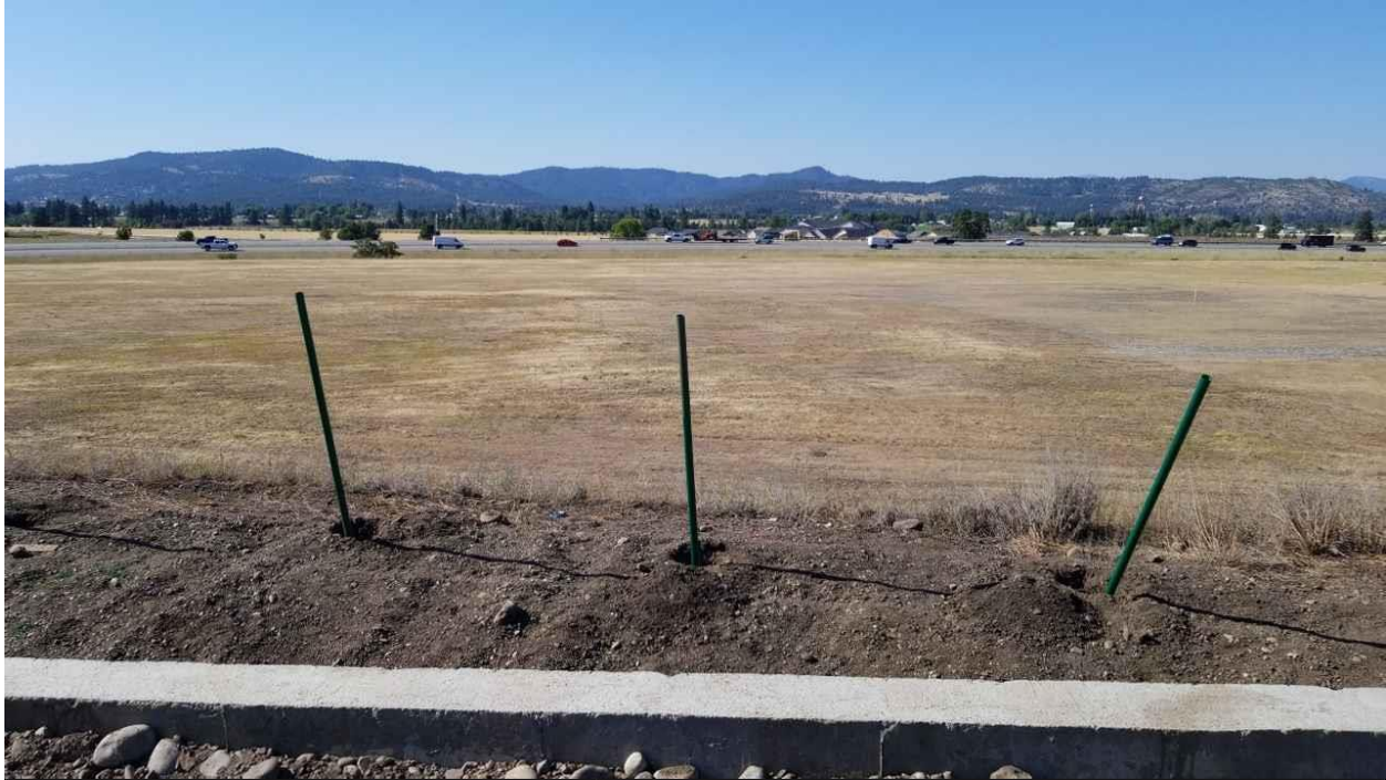
Attachment #5 – 3 Locator's pictures upon his arrival showing that post holes had already been augered
