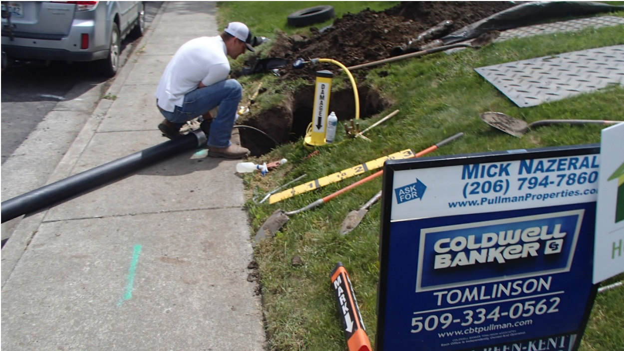
Picture #8 Looking east toward the damage location
