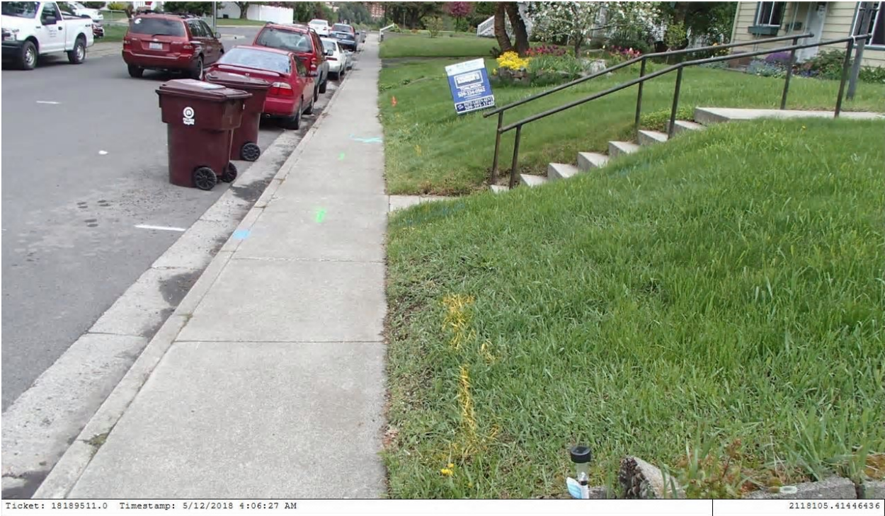
Picture #1 Original locate marks showing the gas pipeline locate marks looking east down the property.
