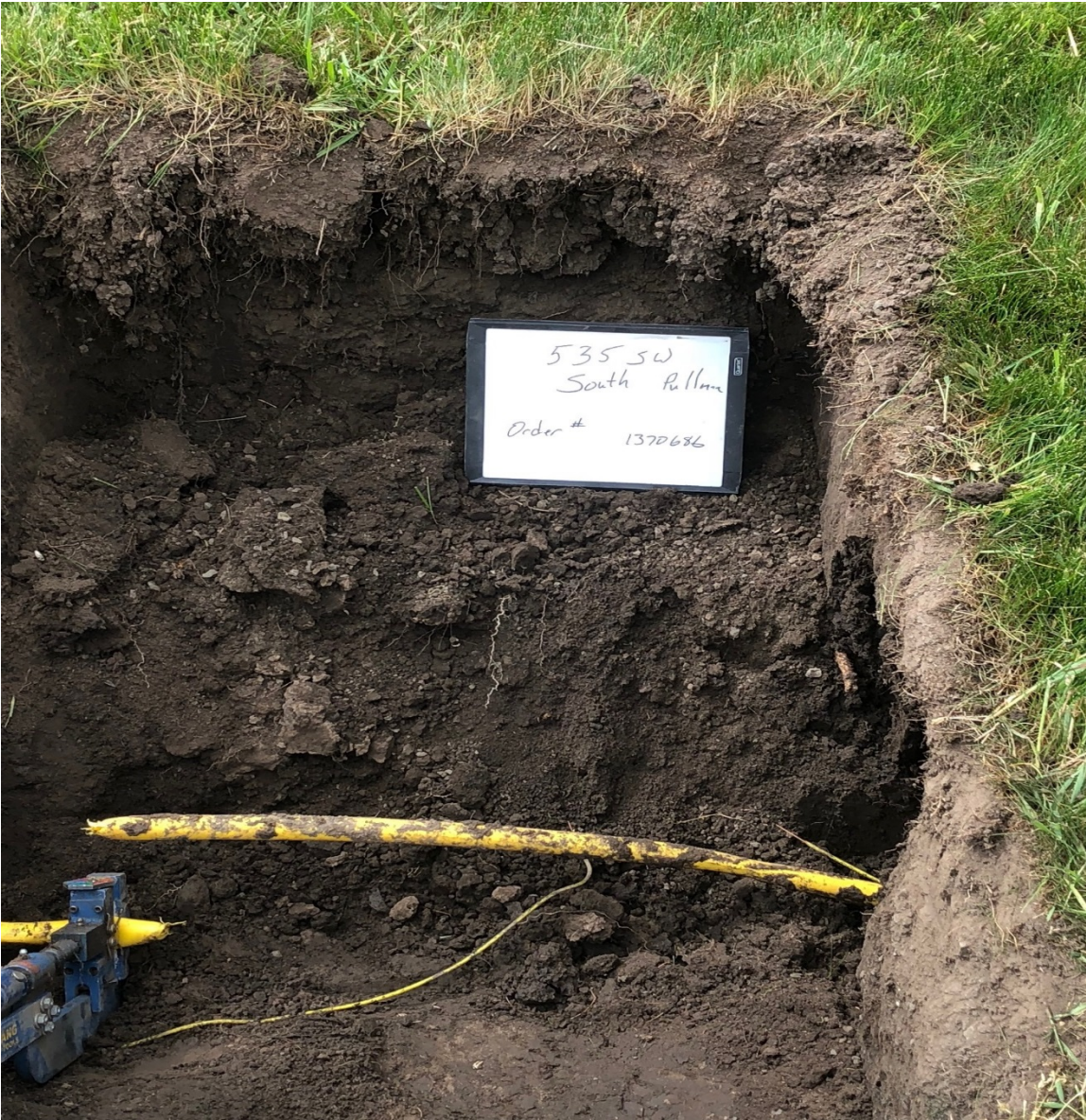
Picture #11 Showing location of damage and trouble order number
