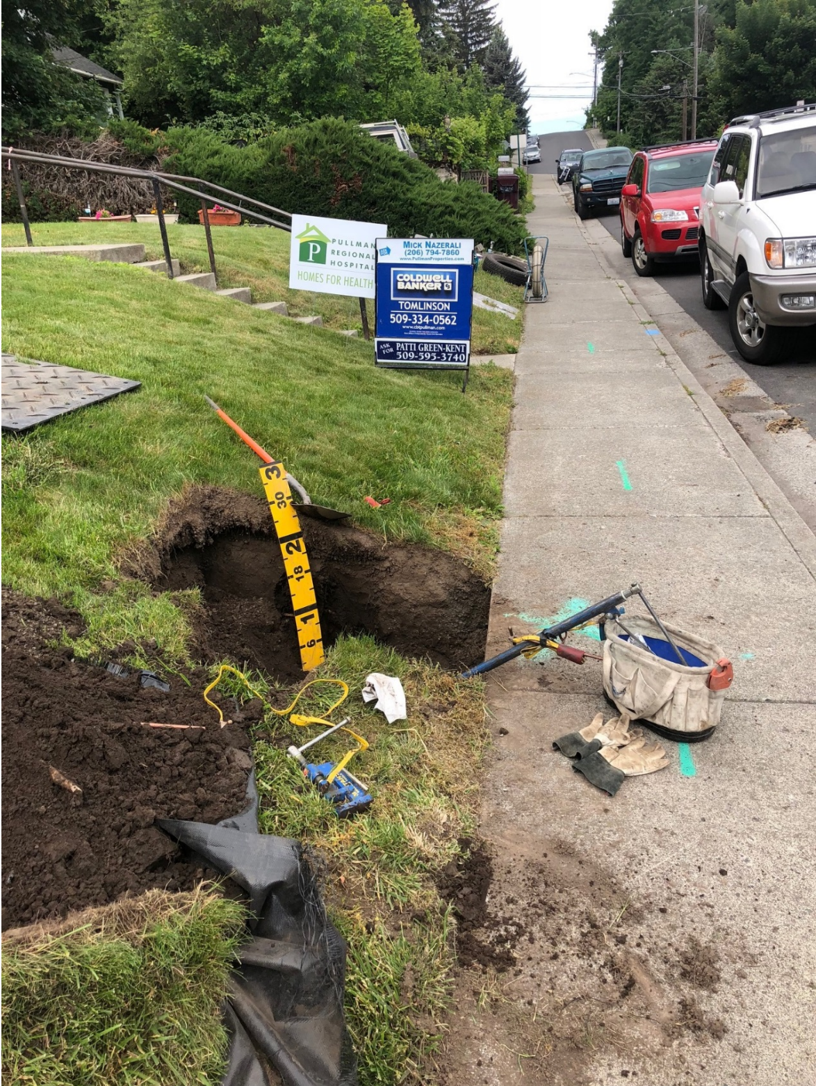
Picture #3 dated 6/4/18 showing where damage occurred. Picture also shows yellow gas line marks faded as compared to Picture #2
