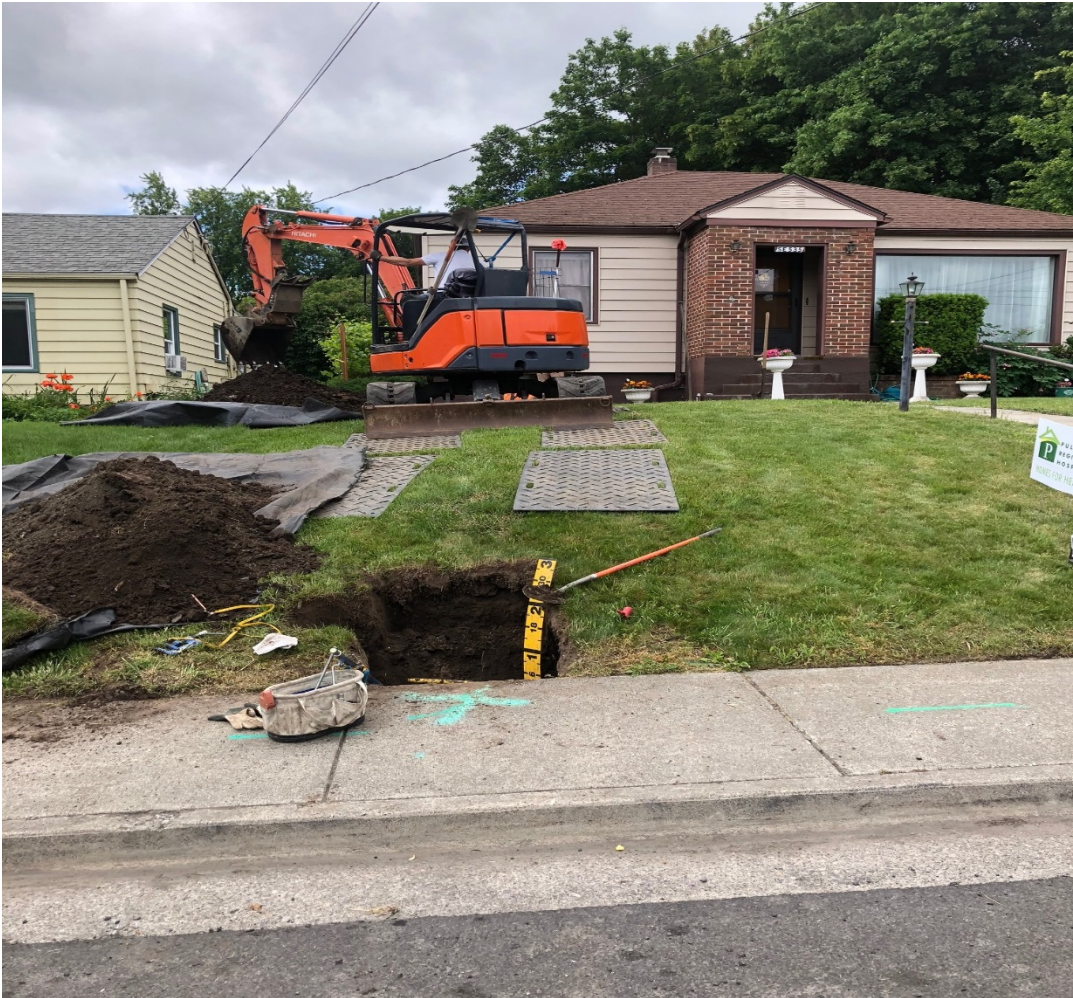
Picture #10 View of damage location looking south towards house.
