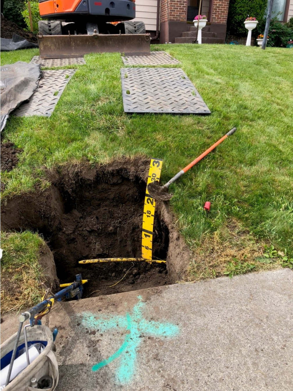
Picture #9 Looking south towards the house at 353 SE South St showing damage to pipe and where backhoe was located at the time of the damage on skid plates.
