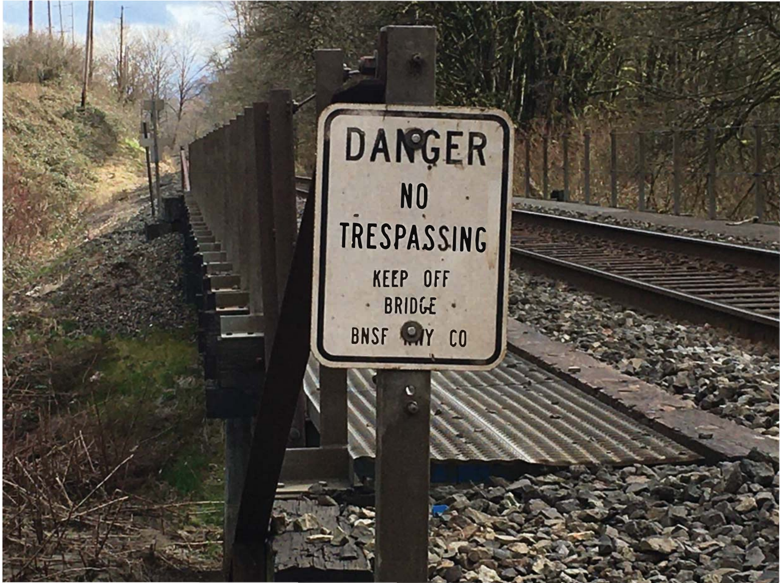
Danger No Trespassing Keep Off Bridge Sign
