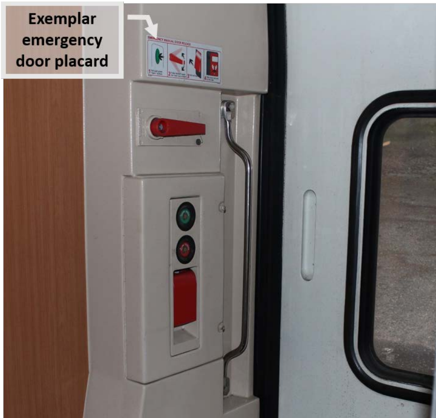
Figure 37. Exemplar emergency door showing instruction placard.
