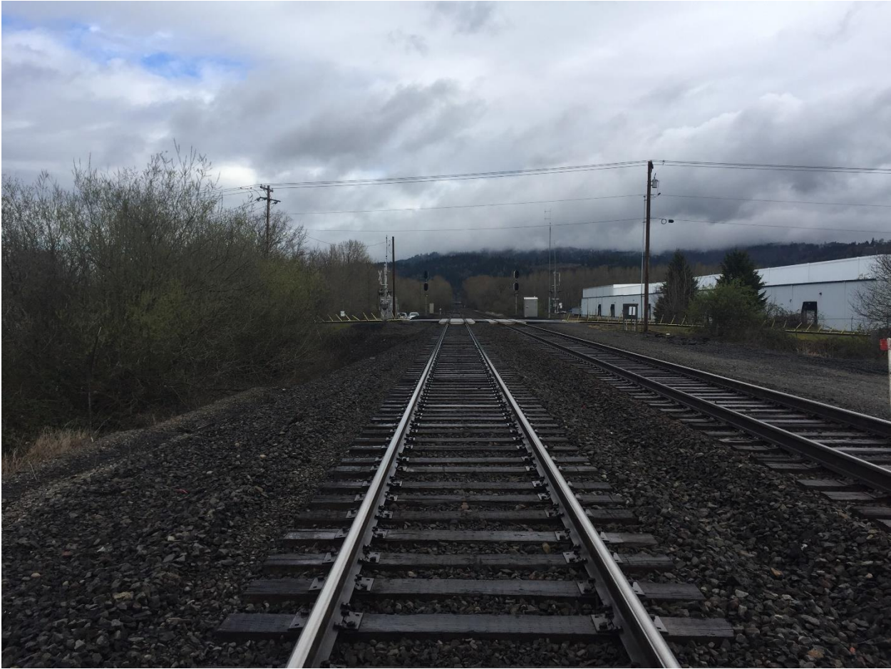
TR-171018 (1) Facing North Toward Accident Site. Photo Taken by Andrew McMahon on 03-23-2020.
