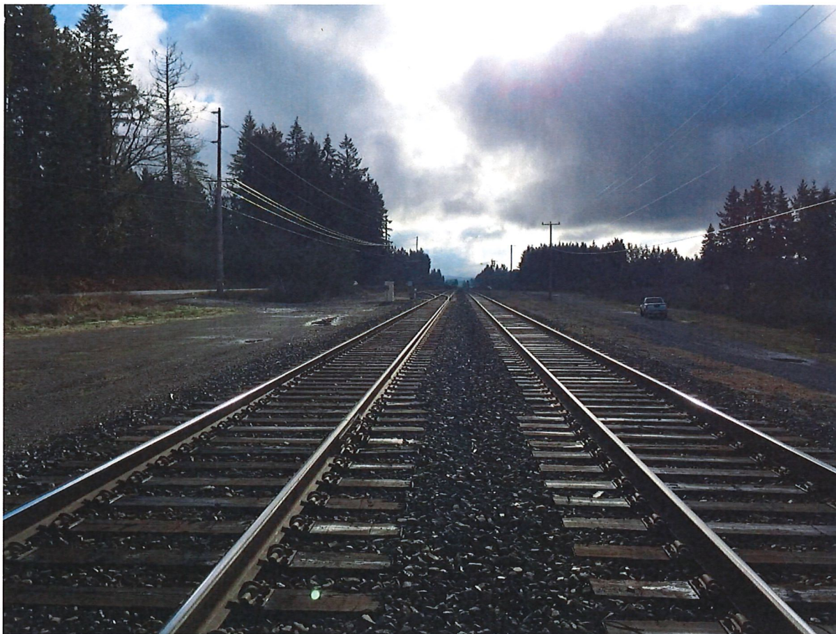
TR-170876 (2) Facing South Toward Accident Site. Photo Taken by Andrew McMahon on 12/27/2018.
