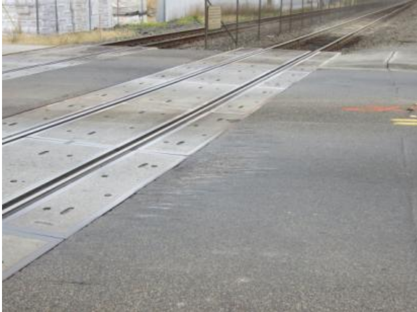
Figure 1 Scrape Marks from Cars Bottoming Out
