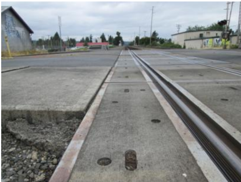
Figure 2 Heaved Asphalt and Uneven Sidewalk
