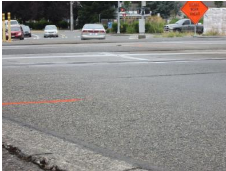
Figure 3 Asphalt Heaved Above Crossing Panels
