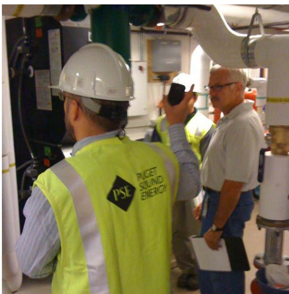
A Verification Team Quality Assurance Specialist verifies a condensing boiler in a multifamily installation.
