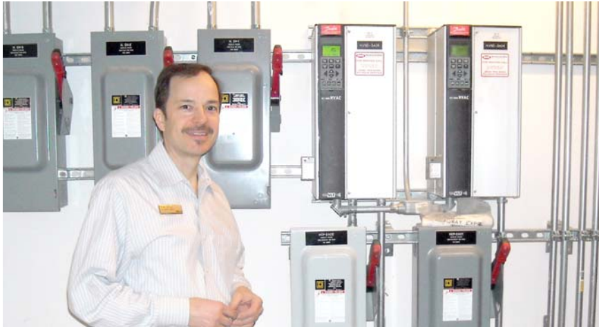
Tim Altier, Chief Engineer, The Westin Bellevue, is pleased with low-cost / no-cost measures like changes in HVAC scheduling.
