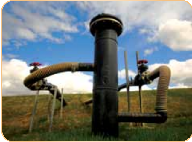
An extraction well collects gas from the landfill and routes it to the new landfill gas-to-energy facility for conversion to marketable natural gas
