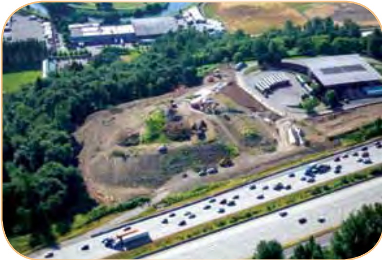
Site preparations are underway for constructing the new Bow Lake Transfer Station on property just north of the existing station.
