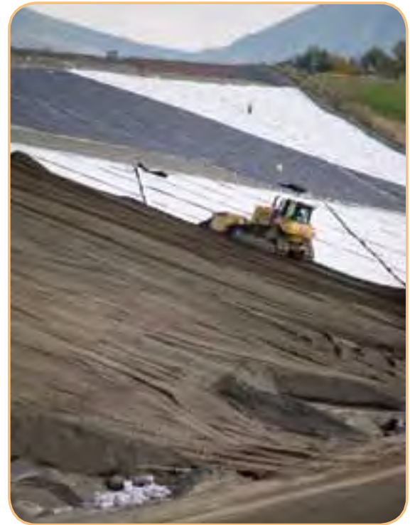
Portions of Area 6 are being prepared for closure with the placement of a soil and geosynthetic layer over the garbage.
