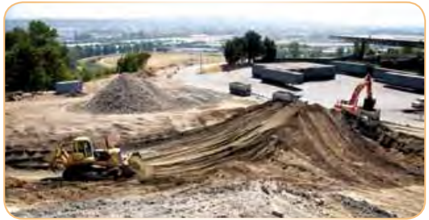
Construction of new transfer stations, such as the Bow Lake station, is financed using general obligation bonds.
