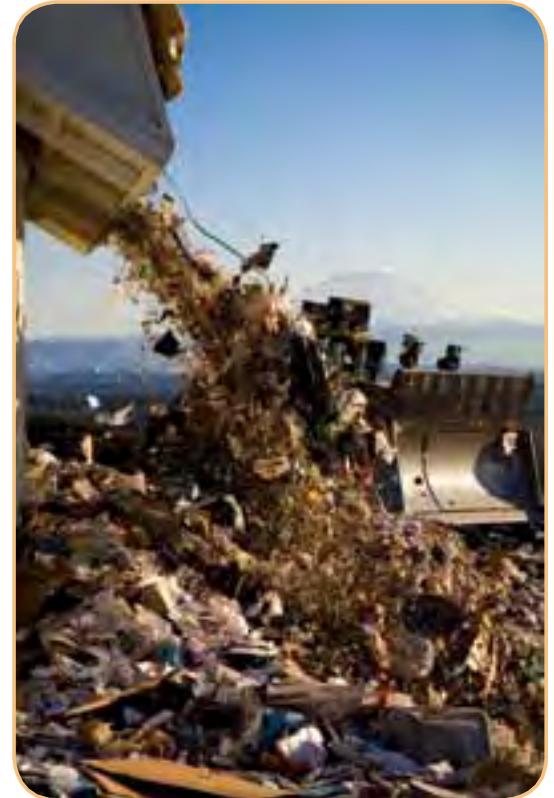
The Cedar Hills Regional Landfill has been in operation since the early 1960s.
