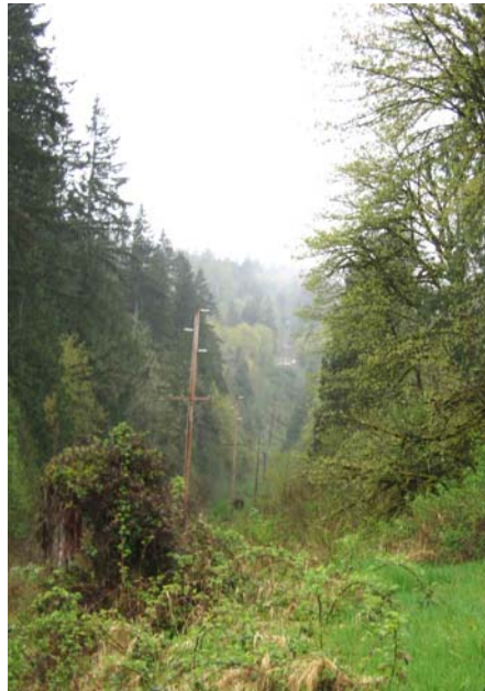
Exhibit 14-4: Vegetation Impeding ROW Access
