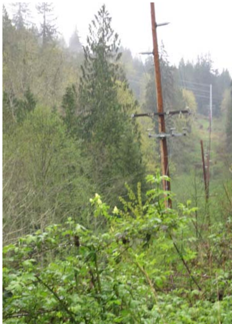
Exhibit 14-5: Vegetation Impeding ROW Access
