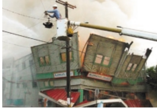
When fire broke out in August 2003 at a landmark building in Port Townsend, our state's historic seaport town, lineman Rick Johnson was quickly at the scene attempting to remove power cables.
