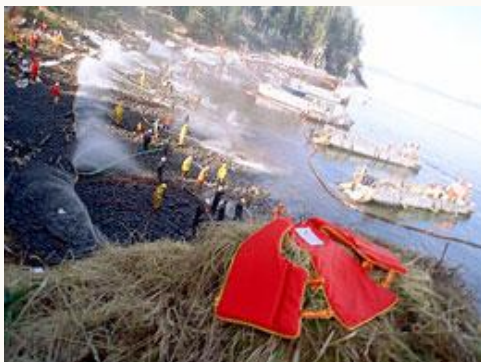
A government-created panel concluded that high-pressure hoses used on Prince William Sound beaches during the cleanup did more harm than good. WIKIMEDIA
