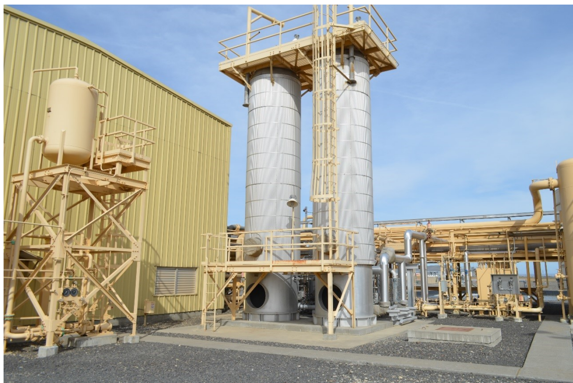
LNG-2 Adsorbers – undamaged – identical to LNG-1 adsorbers pre-event.
