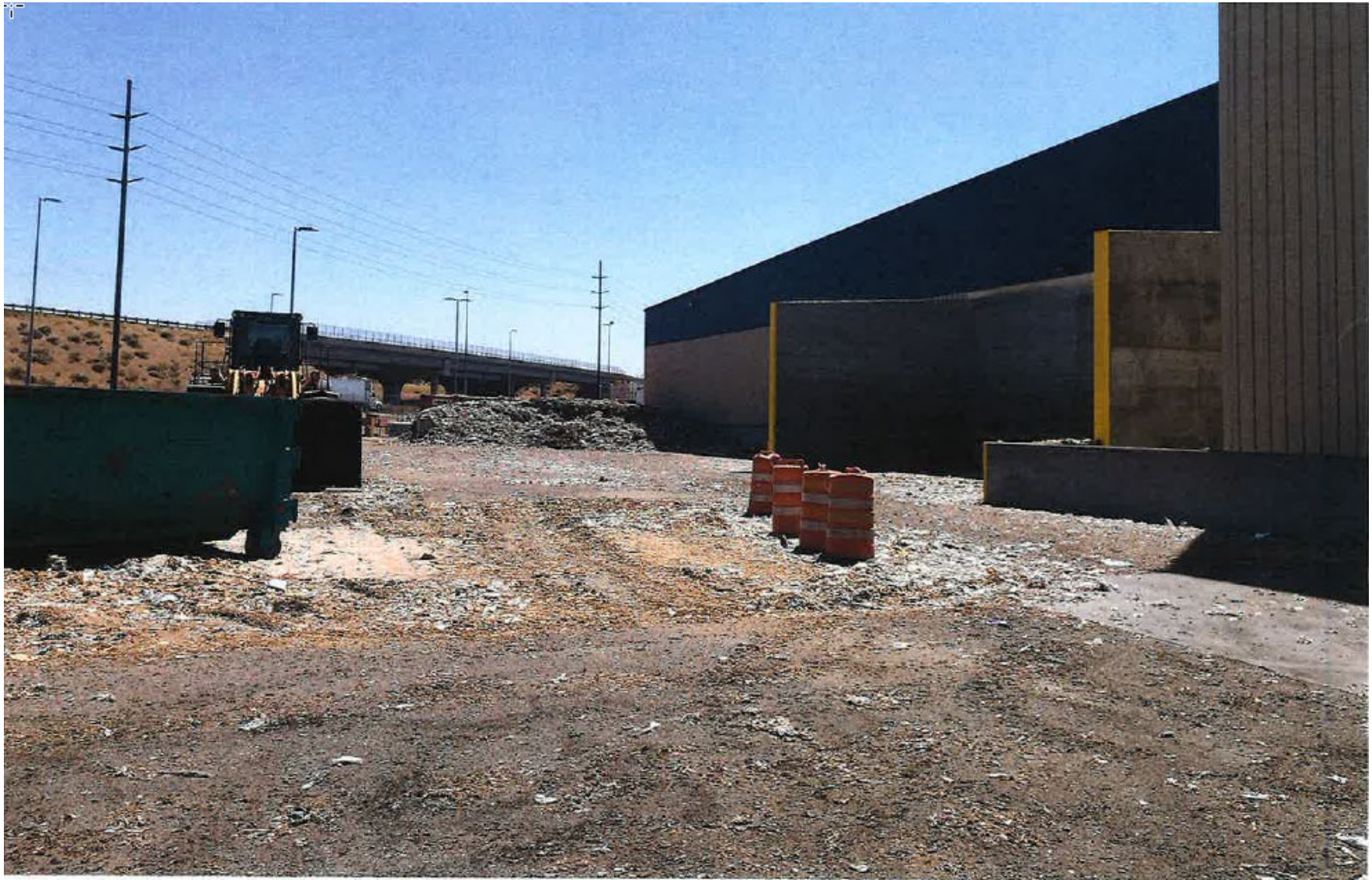
Jammies eliminated piles in front of building and are managing under a concrete bunker.
