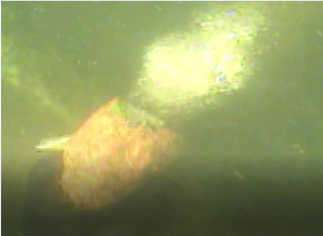
Figure 8- Diffuser #3 during flow test
