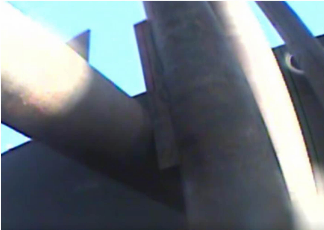
Figure 10- Above water of 8" pipe welded to horizontal support
