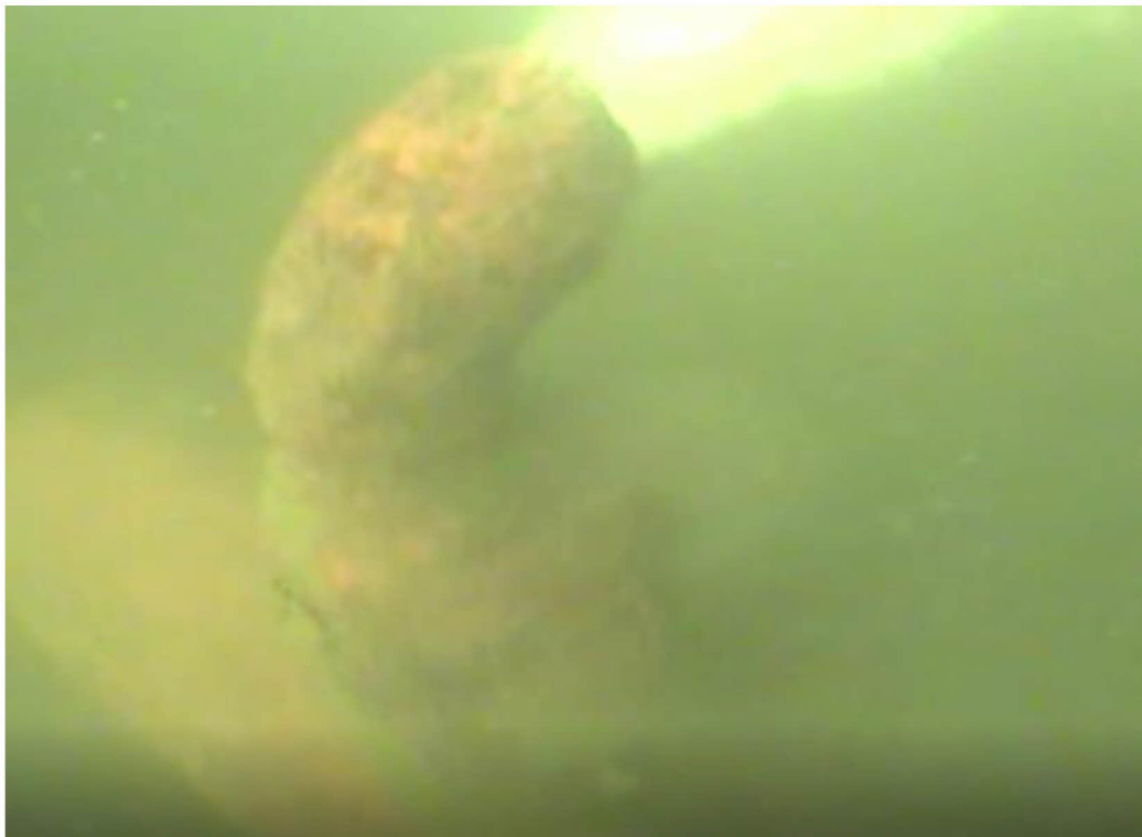
Figure 7- Diffuser #2 during flow test
