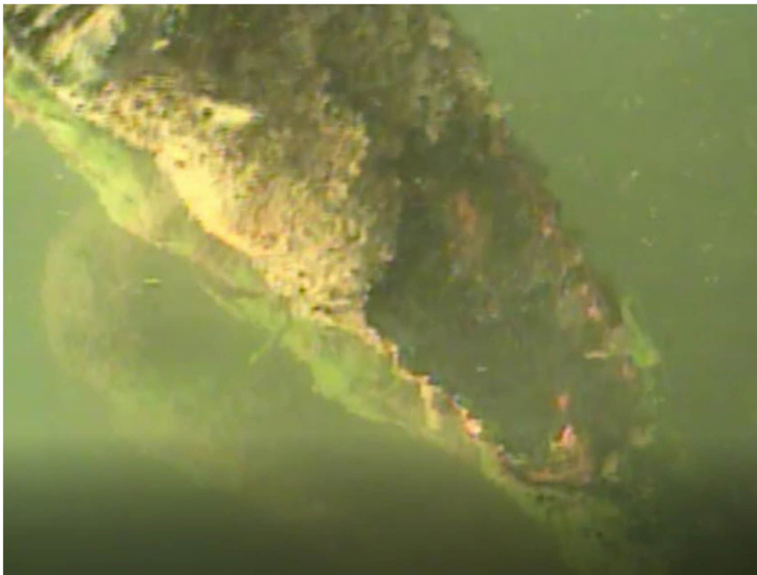
Figure 11- Below water vertical support with marine growth, rust build up and clean area exposing pitting
