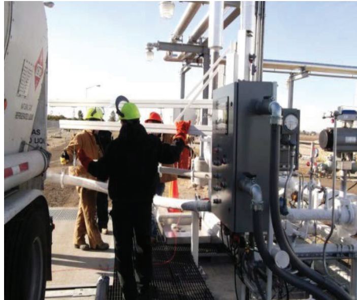
Figure 10 – Example LNG Truck Tanker Loading Operation
