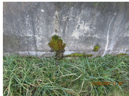
North Side Large Storage Tank
