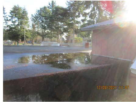
Large Storage Tank - Ponding
