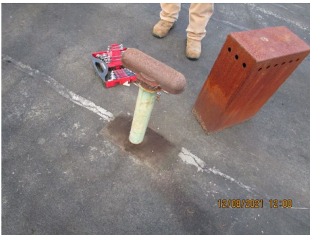
Large Storage Tank Vent
