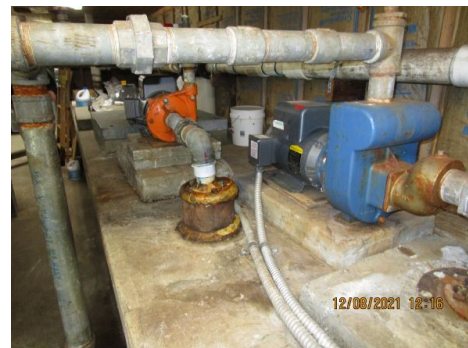
Booster Pumps for Small Storage Tank
