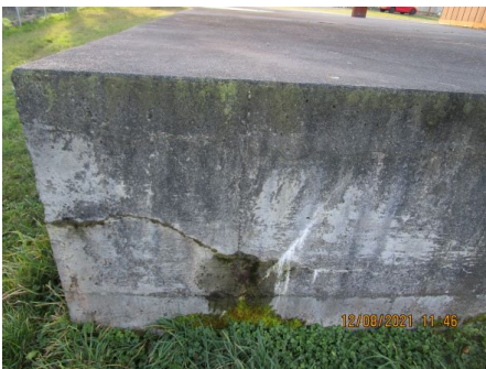
North Side Large Storage Tank
