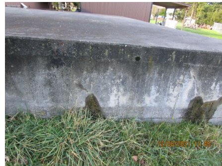
East Side Large Storage Tank
