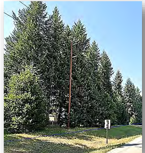
CDA-Rathdrum 115 kV along US Hwy 95
