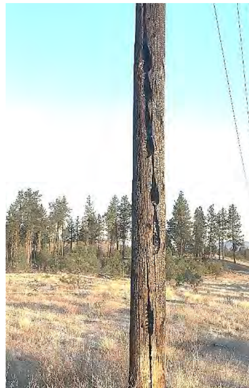
Pole fires generally occur on wood poles with wood crossarms. Since the early 2000's, Avista has adopted fiberglass crossarms as the standard unit. Replacing wood crossarms in elevated fire risk areas is a component of Wildfire Resiliency.
