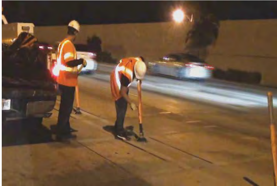
Figure 3. Sheeting Failure and Post Failure Replacement.
