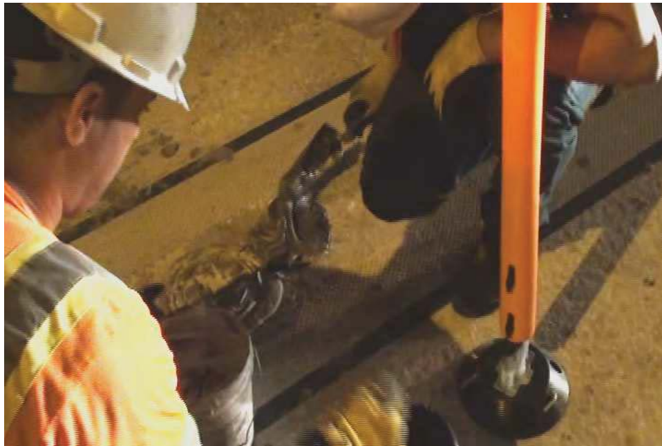
Figure 5. Epoxy Failure and Pavement Failure Replacement.
