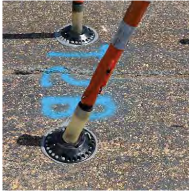
Figure A-4. Sample 2B Failure at 44 Impacts.
