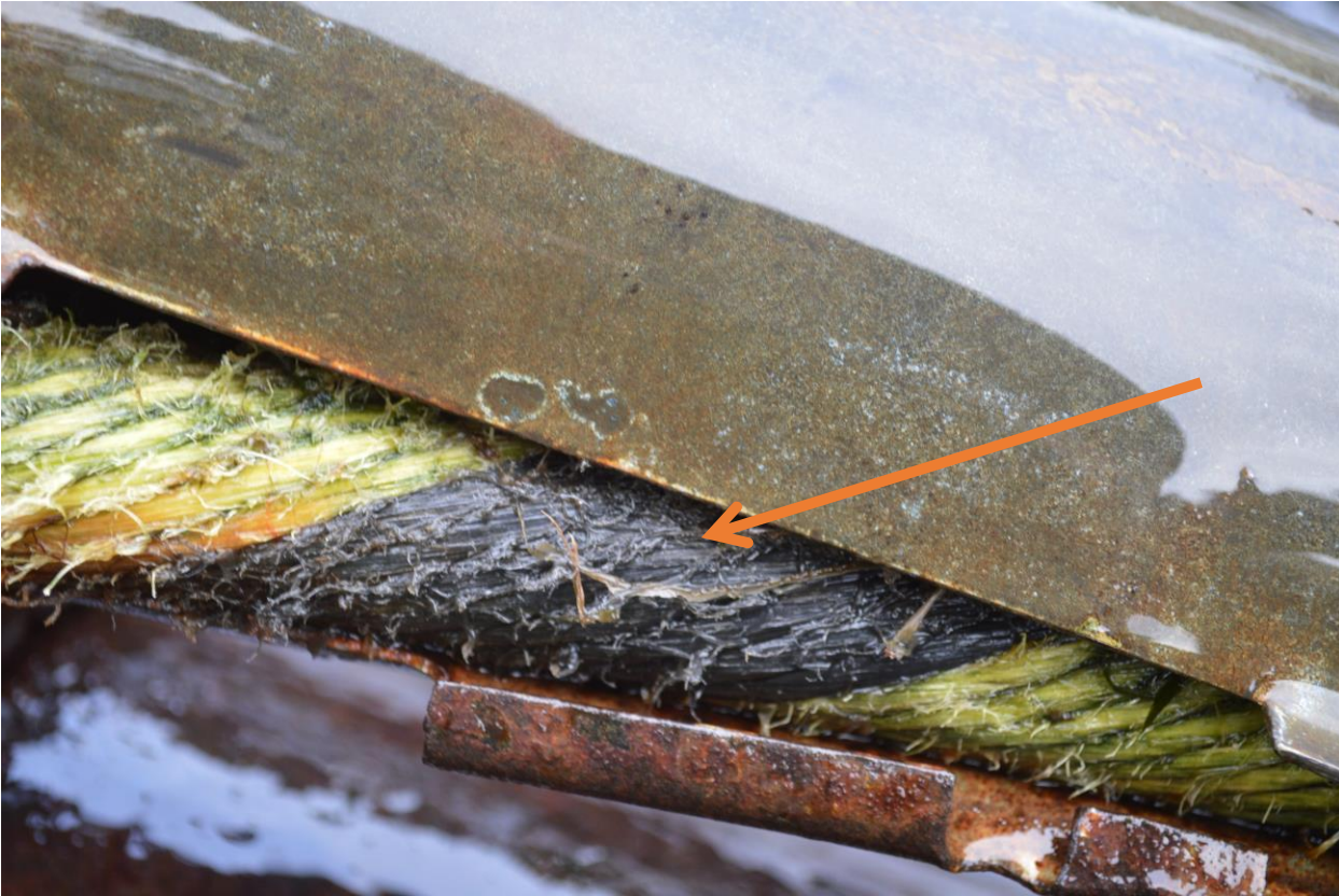
Exhibit 5 CenturyLink Fiber Optic Cable Exposed 3
