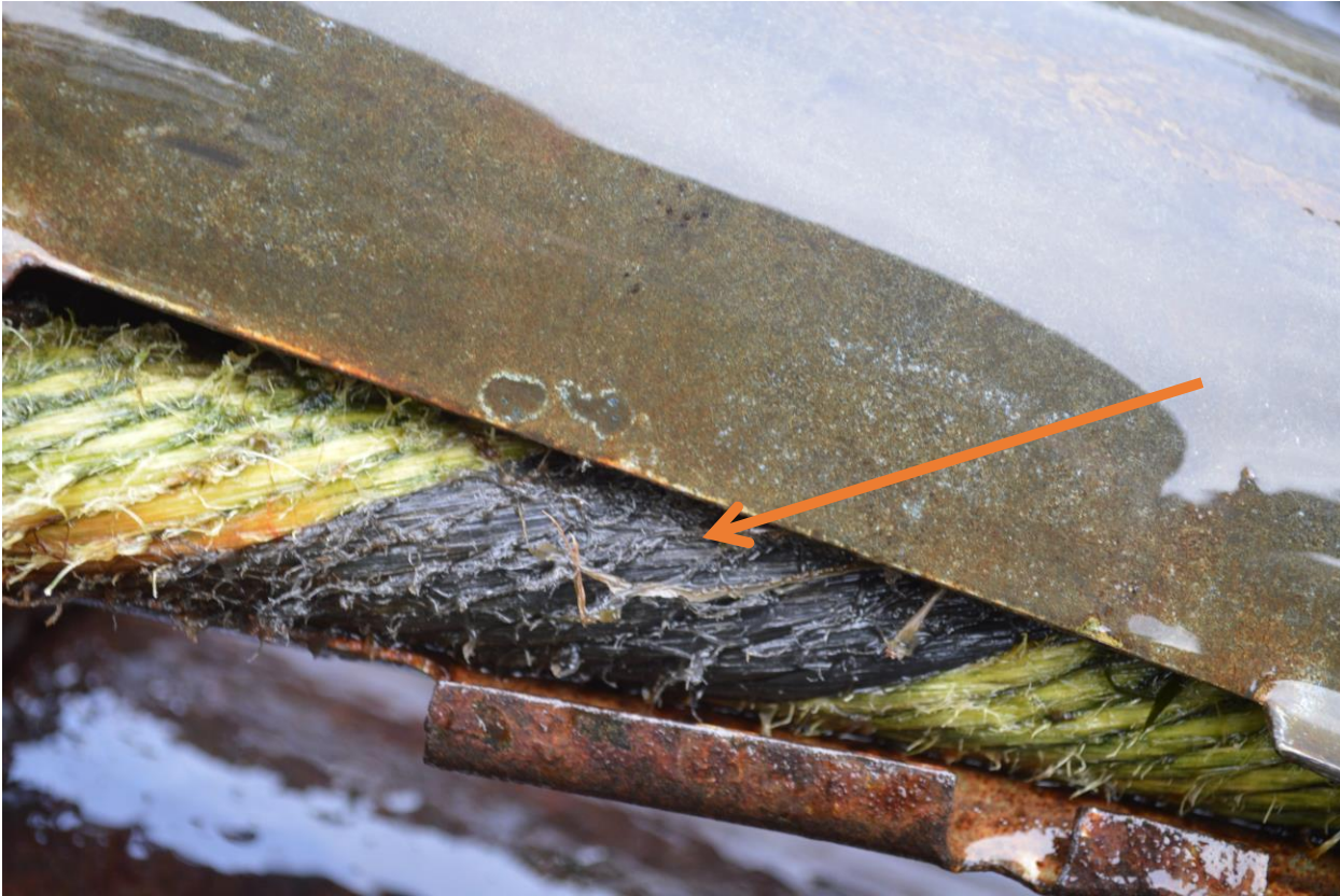
Exhibit 5 CenturyLink Fiber Optic Cable Exposed 3
