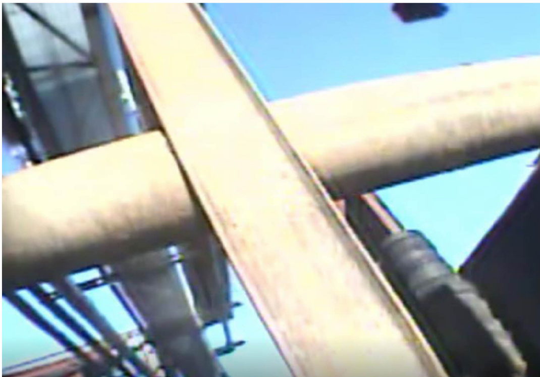
Figure 7 - Above water view of vertical channel support welded into horizontal support
