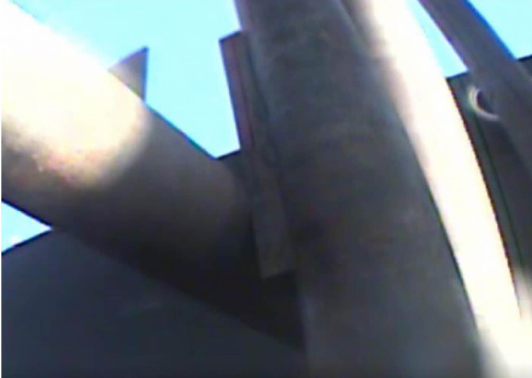
Figure 6 - Above water of 8" pipe welded to horizontal support
