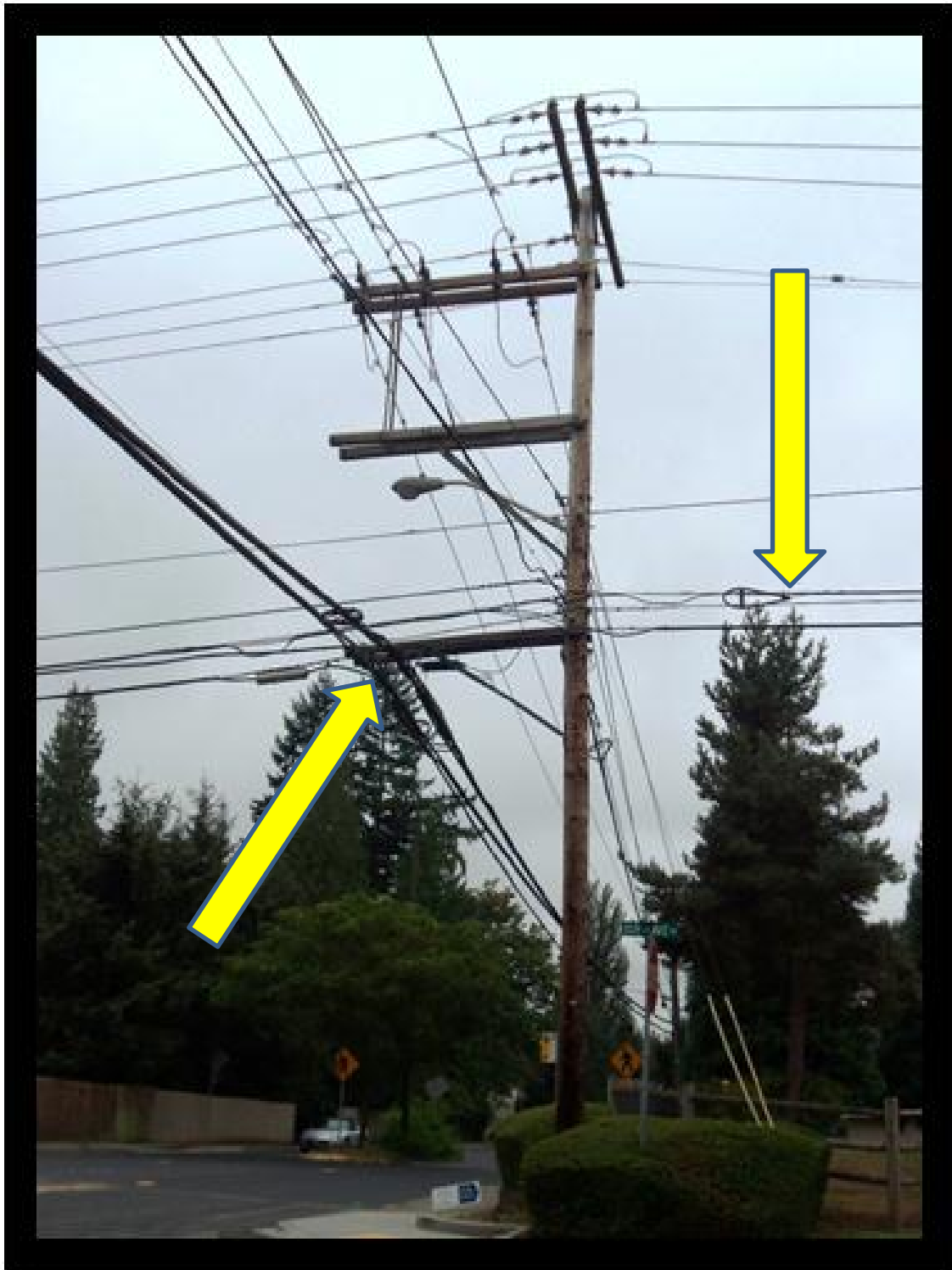
Figure 2. Note amount of overlashing and size of overlashed conductor bundles and installation of stand-off bracket and the impact on the pole.
