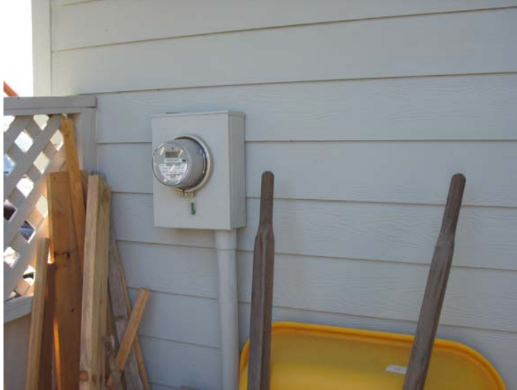
Figure 3.4. GoodWatts™ Energy Meter, as Installed by Trained Utility Electricians
