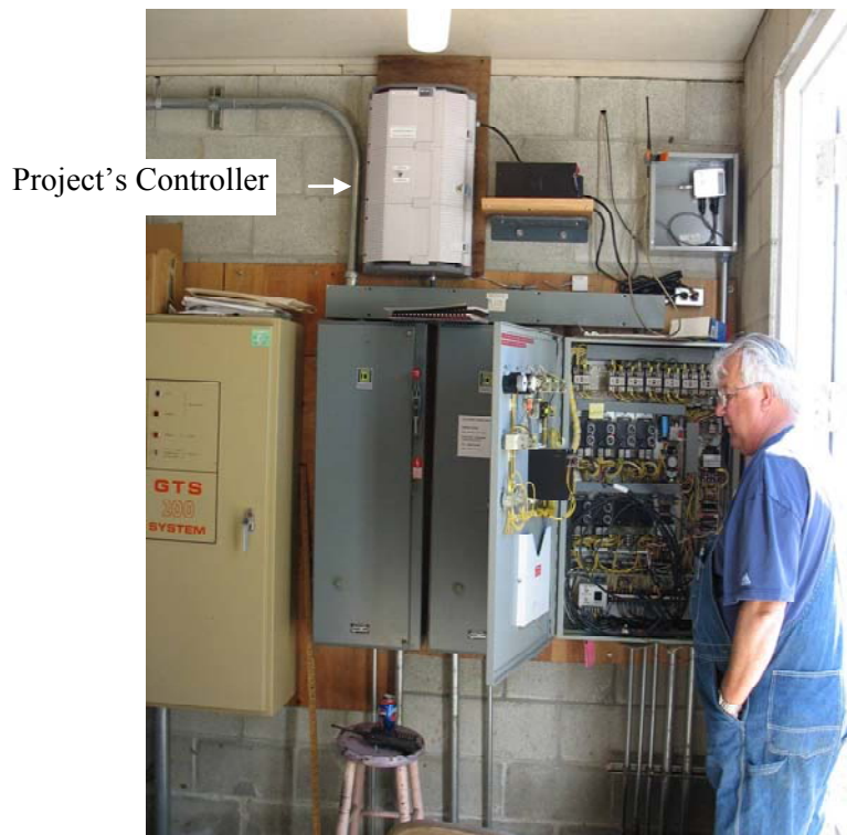
Figure 5.4. Control Panels at the Sekiu Pumping Station
