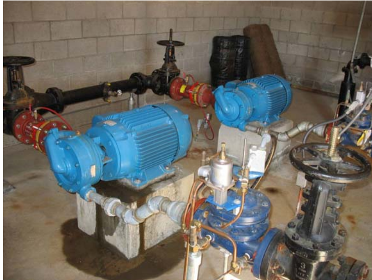
Figure 5.1. Pumps at the Sekiu Water Pumping Station
