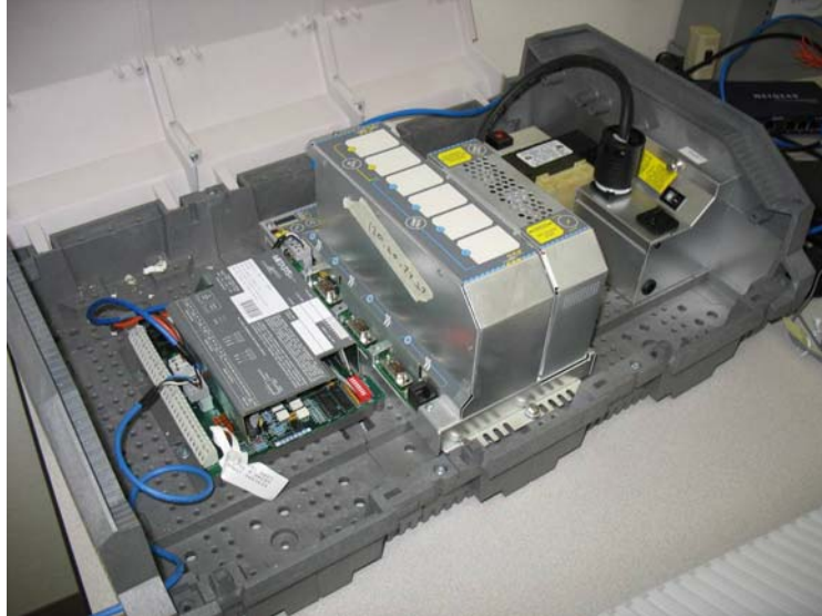
Figure 5.5. Pump Controller Hardware
