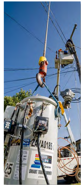
Avista “Smart” Transformer
