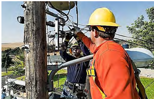
Upgrading the Distribution System in Pullman Phys.Org, June 10, 2015, https://phys.org/news/2015-07-nation-largest-smart-grid-demo.html
