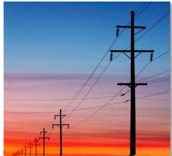
Transmission Poles showing distribution lines “underbuilt” below the transmission lines, which puts additional strain and wear on the poles
