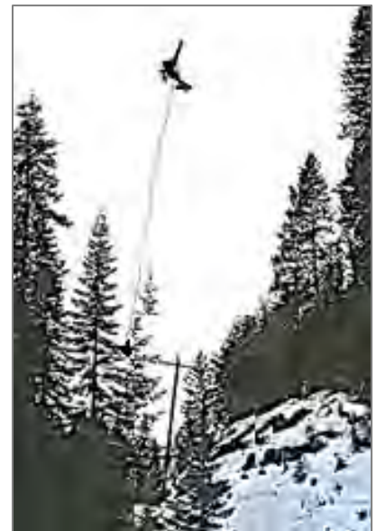
Grangeville's terrain presents some major challenges. At times helicopters must be used to access lines.
