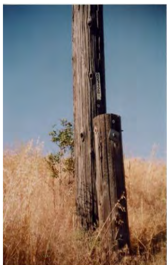
Stubbing a pole can add an additional 20 years or so to the life of a pole
