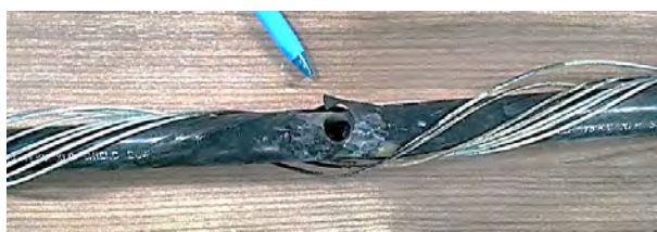
Old cable, susceptible to failure
