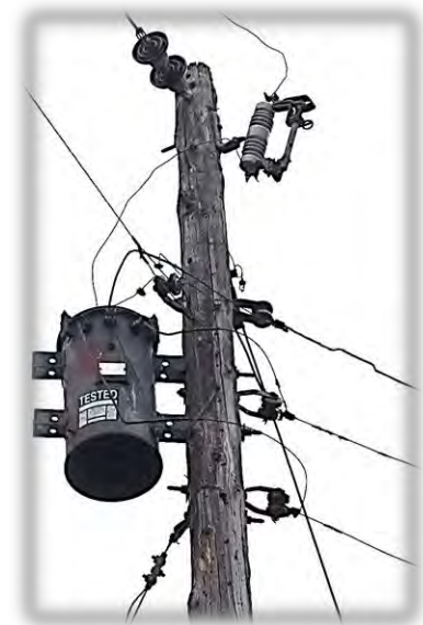
Old equipment increases reliability risk
