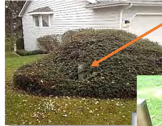
Left: Transformer Covered by Shrubbery
