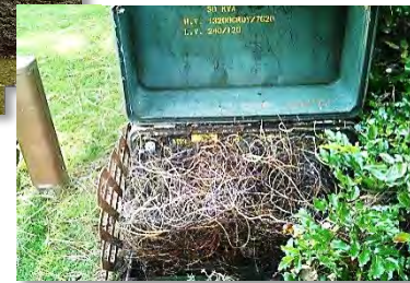
Below: Vines Growing Inside a Transformer Box
