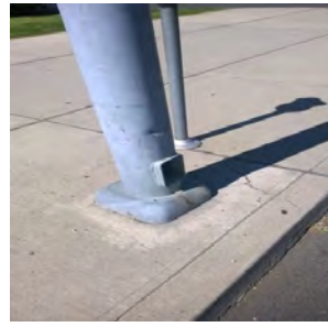
Figure 18: Cracked Concrete, No Cover Missing, Ding
