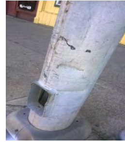
Figure 20: Rust, No Cover, Damage
