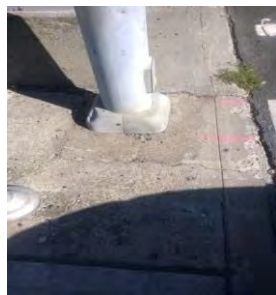
Figure 23: Cracked Concrete, Ding
