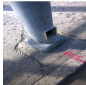
Figure 22: Cracked Concrete, No Cover
