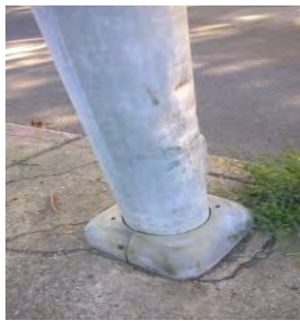
Figure 21: Cracked Concrete, Damage, Rust
