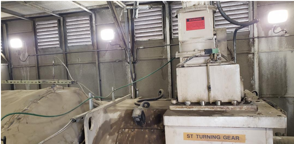
Figure 5: Unit 1 Steam Turbine Building LED Lighting
