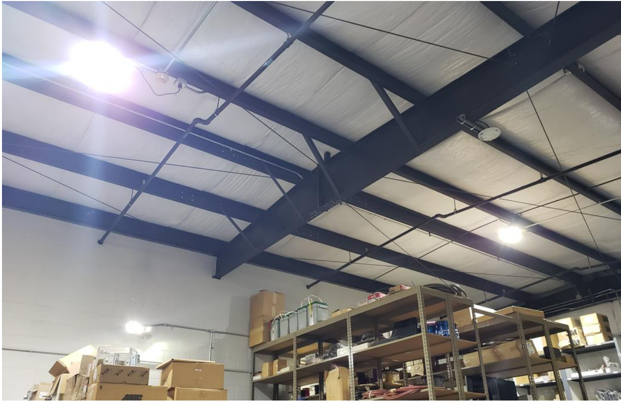
Figure 4: Maintenance Building LED Lighting with Occupancy Sensors
