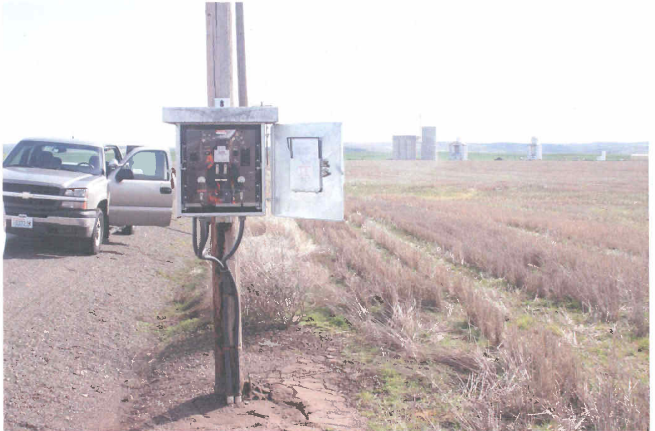
TransCanada Pipeline, Wallula District MP 224.2 Clyde Rectifier Babcock Road Universal Rectifier Inc. Model: ASAI Serial #: 103057 Photo taken by: Al Jones 3/16/2011
