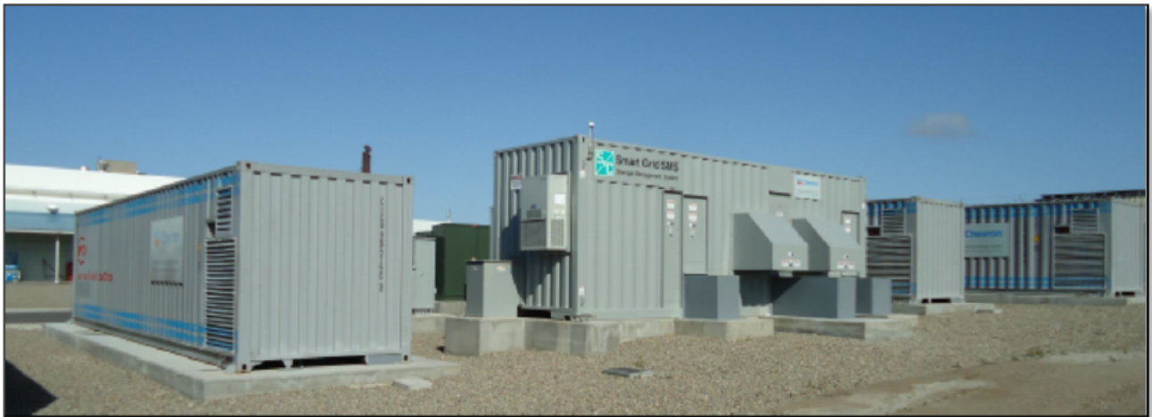
Figure 2: Example 2MW/4MWh BYD system provided for Chevron, Santa Rita, CA
