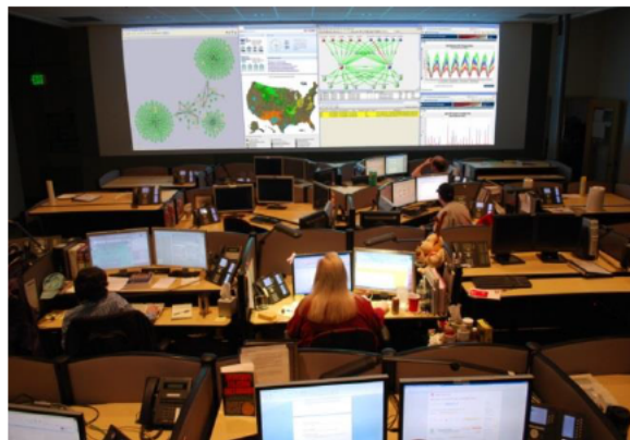
Exhibit 125. TCS Network Operations Center
