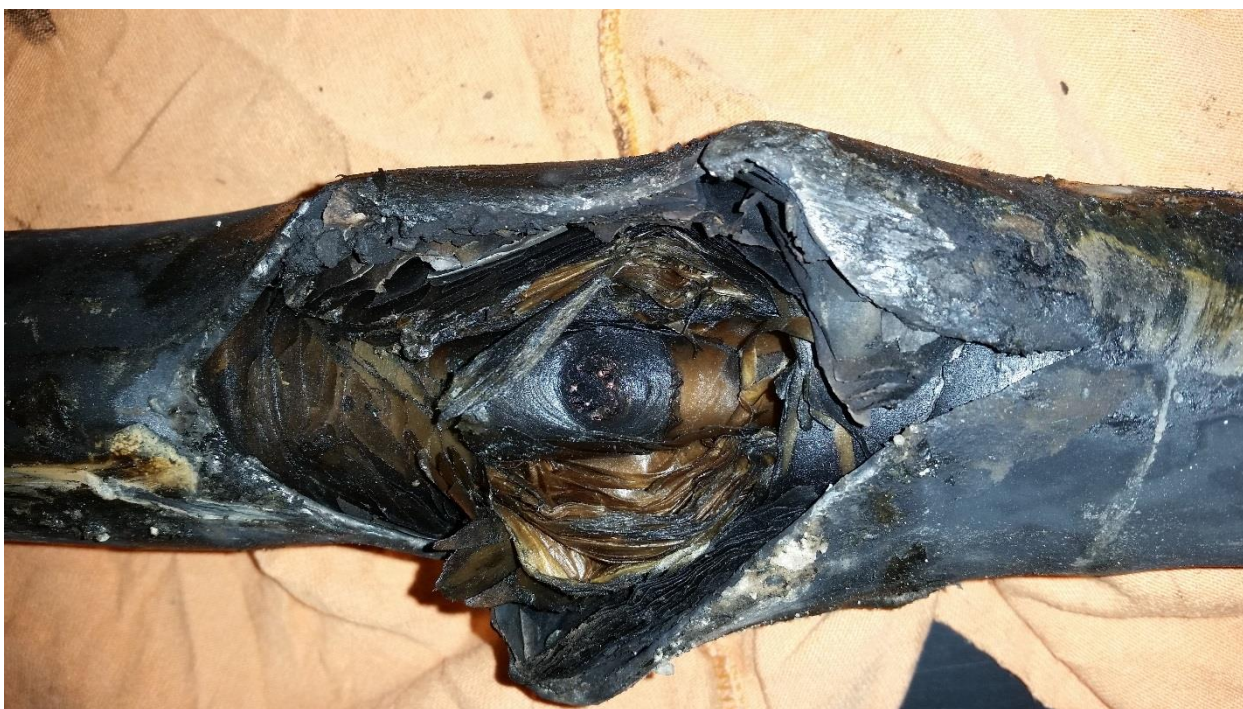
Figure 22, A faulted PILC cable
