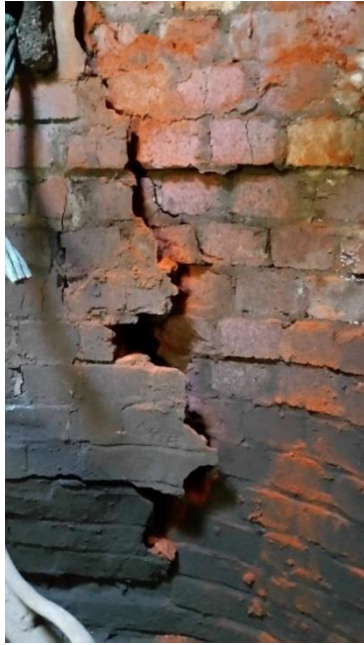
Figure 25, Interior of a badly deteriorated old manhole in a heavily traveled street
