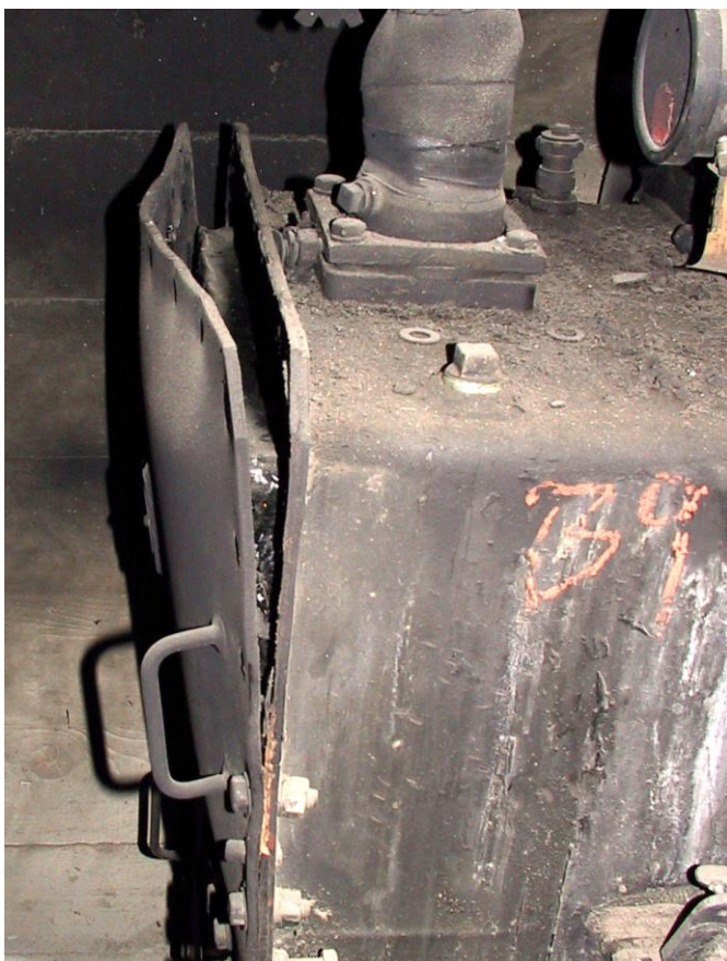
Figure 24, A network transformer after a failure in the primary compartment
