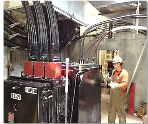
Downtown Network Vault
