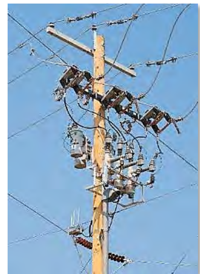
Figure 20. Dry Land Mode Device: Viper Recloser
