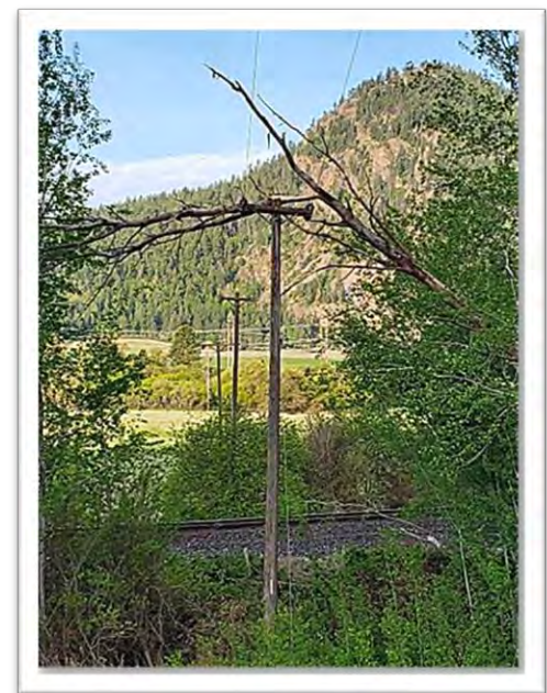
Figure 16. Dead tree falls into powerline
