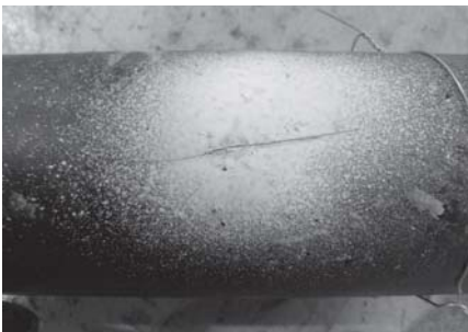
Cause Code E: Rock Impingement or Crack on DuPont Pipe
