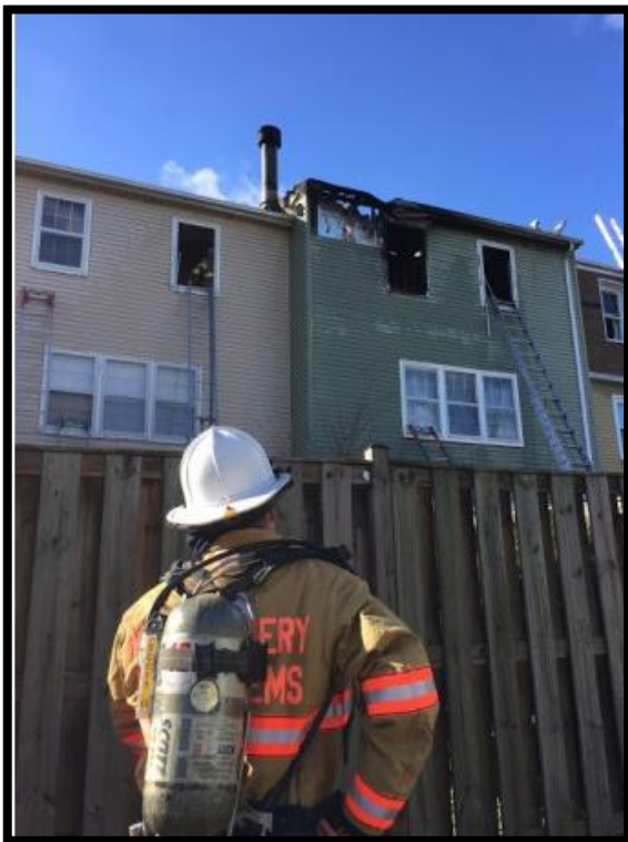
Aftermath of a space heater fire in Prince George's County, MD Source: http://patch.com/maryland/bowie/space-heaters-cause-bedroom-fires-twice-week-0
