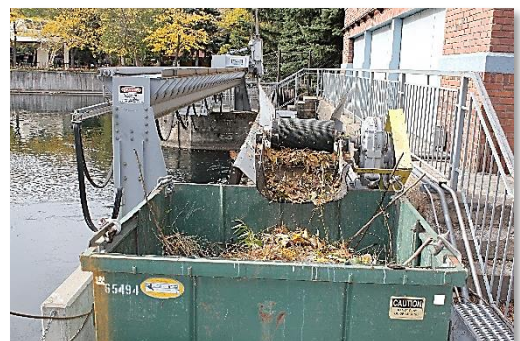
Below: trash rake conveyor system removing the debris
