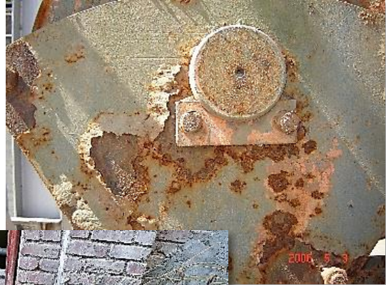
Above: Cabinet Gorge Unit #1 headgate issues
