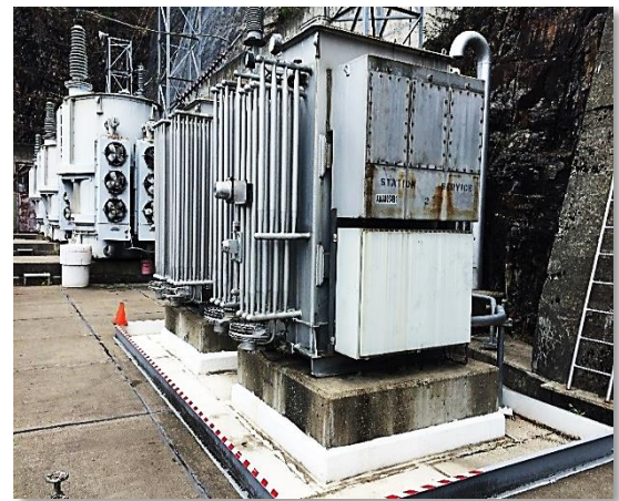
Cabinet Gorge Station Service
