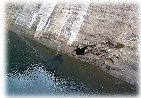
Long Lake Dam erosion
