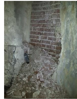
Post Falls wall erosion
