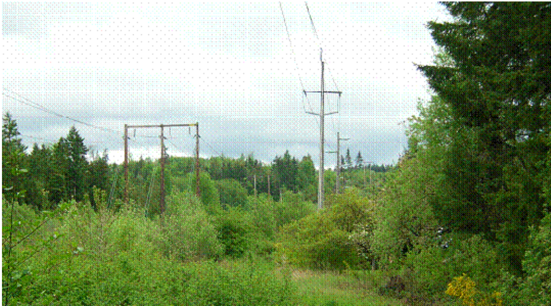
Figure 2-5. PSE (left side) and Clallam County (right side) 115,000-volt transmission lines near PSE's Irondale substation.
