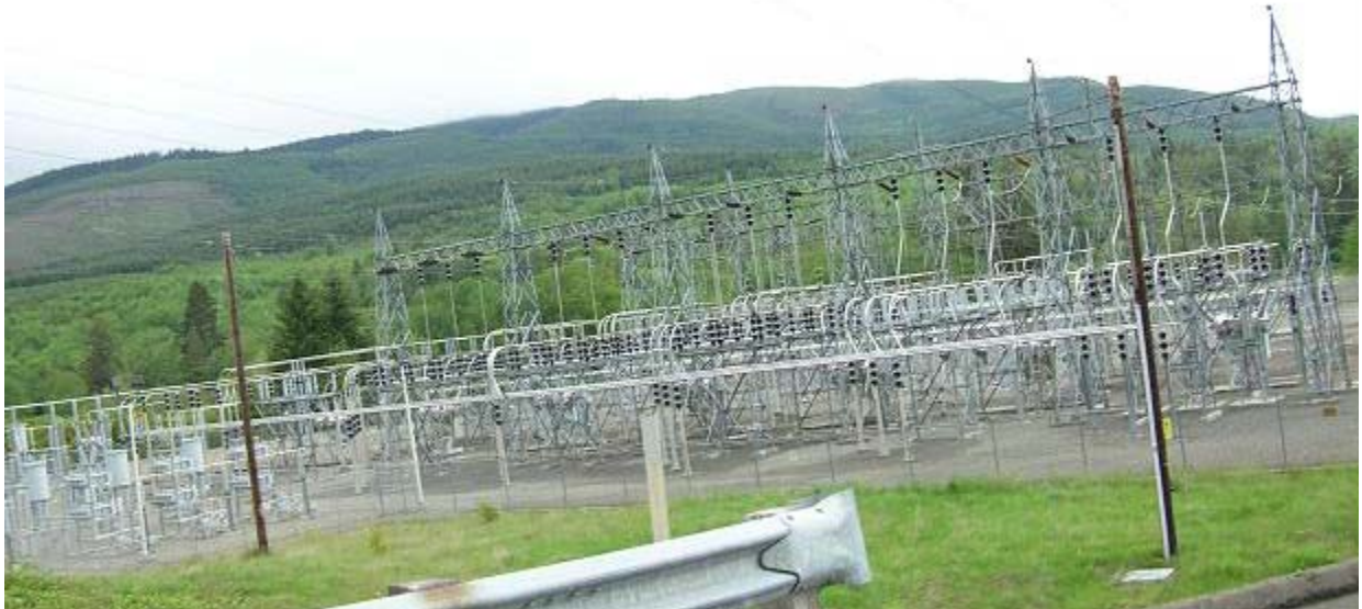
Figure 2-4. BPA's Fairmount Substation.
