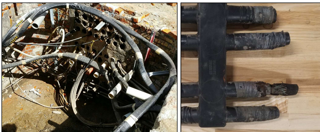
Figure 2: Brick handhole w/assortment of PILC cable / Failed insulation on grid bus (Hotel Ruby Service)
