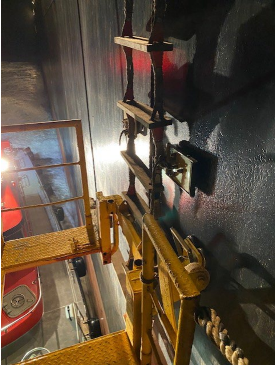
Photograph No. 5 shows ladder ropes resting on the sharp edge of the ship's hull with no chafing gear:
