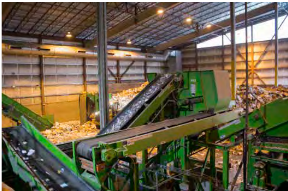
Recology CleanScapes materials recovery facility
