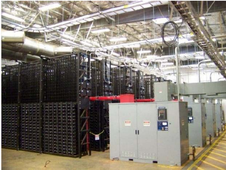
Figure 13 - PowerCell™ Stacks with PCS
