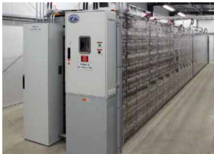
Figure 18 - UberBattery Energy Block
