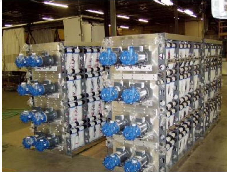
Figure 15 - ZnBr Cell Stacks
