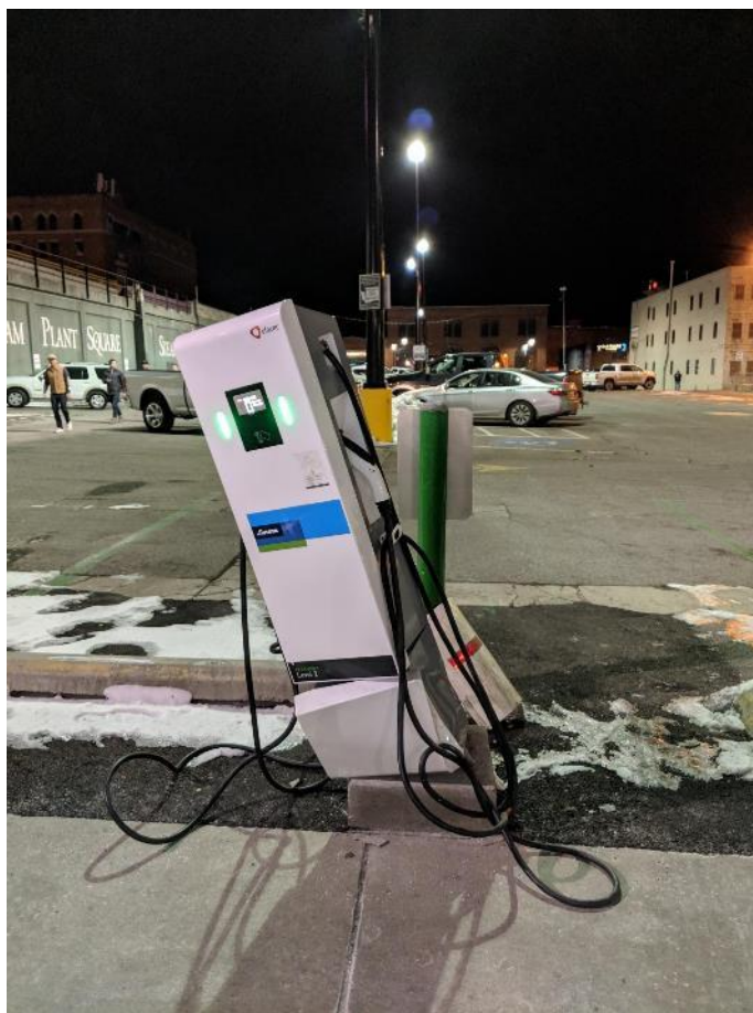
Figure 31. EVSE damage from a vehicle impact
