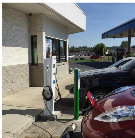
Figure 24: Public EVSE installation
